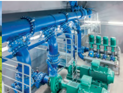
Kapinci-Vaška irrigation system, pumping station
